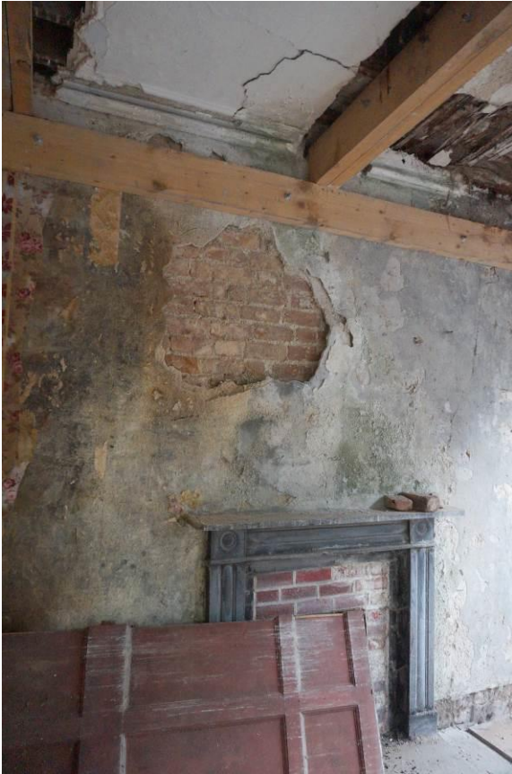
Fig. 3: Propped floor, ceiling over first floor.
