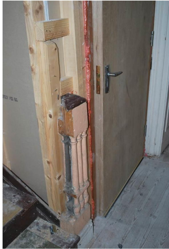
Fig. 4: Lobby inserted to stair landing and damaged balustrade.
