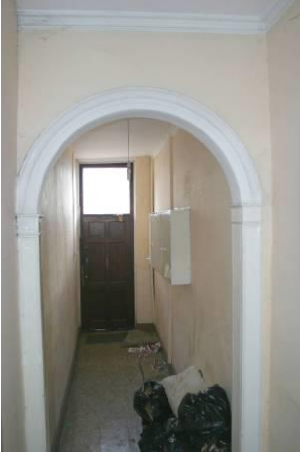
View from bottom of the staircase to front door, showing front hall, architrave to arched opening and cornice to ceiling.
