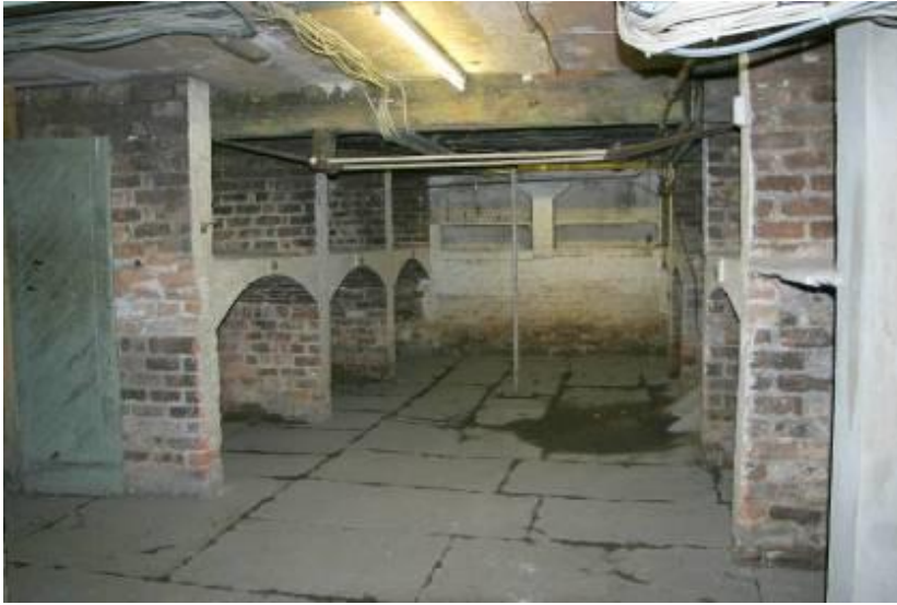
Area to the front of 9 Ellen Street, showing the flagged floor and the brick wine storage units.
