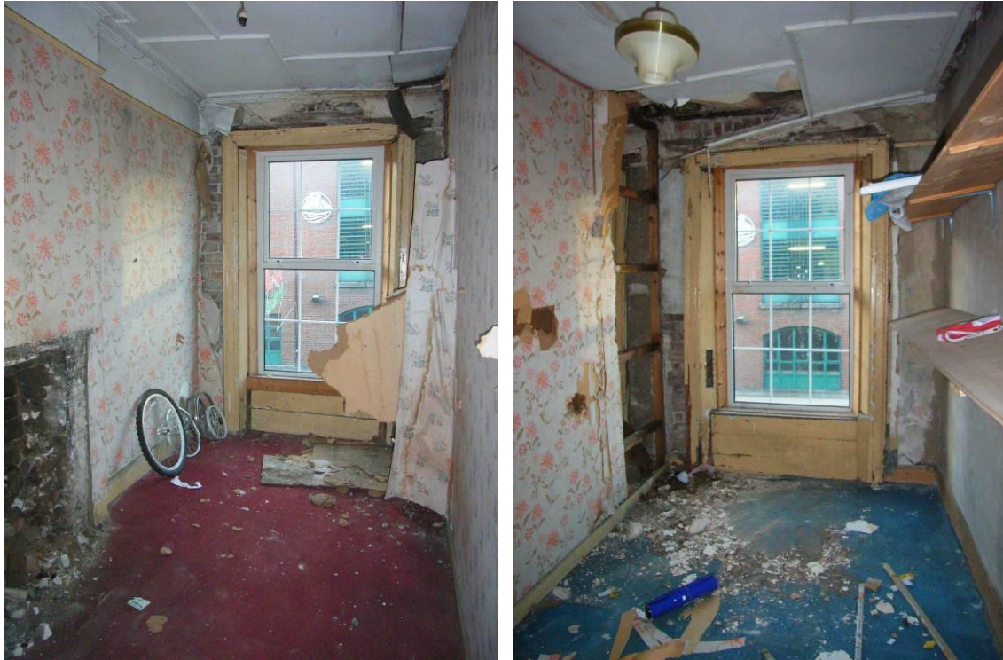
View of front room (partition wall to the middle), showing the fireplace with fire surround removed and the timber architraves.
