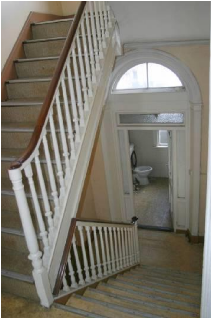
View of staircase showing round-headed opening to the half landing between ground and first floor levels, which was originally a window opening.
