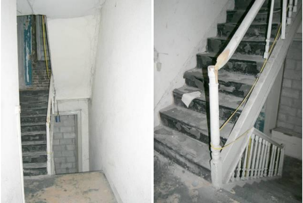
General view of staircase between second and third floors (above left) and detail showing balustrade (above right).
