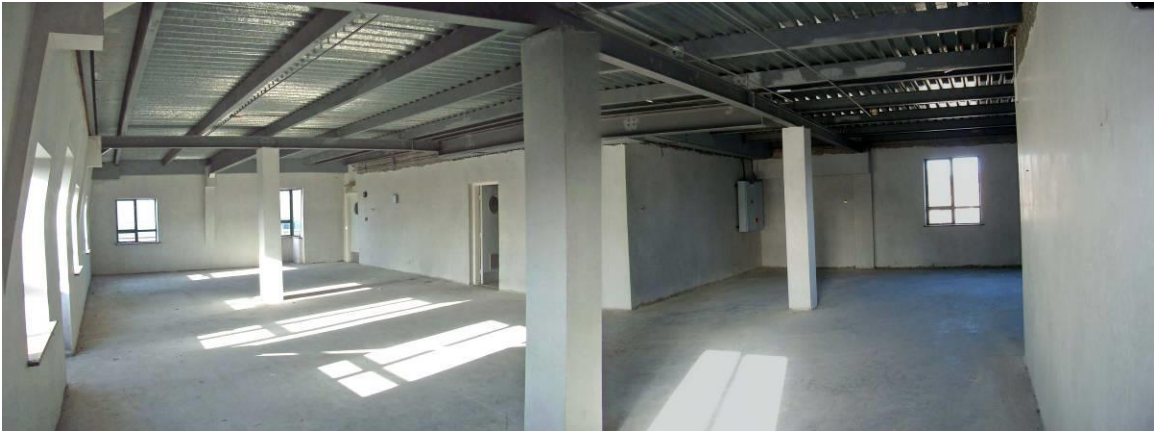
Forth Floor showing Metal Roof – note also no raised access floor indicating possible previous use for storage only.
