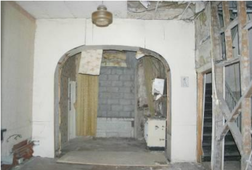
View from rear room to rear of building, showing original rear wall and blocked up window opening.
