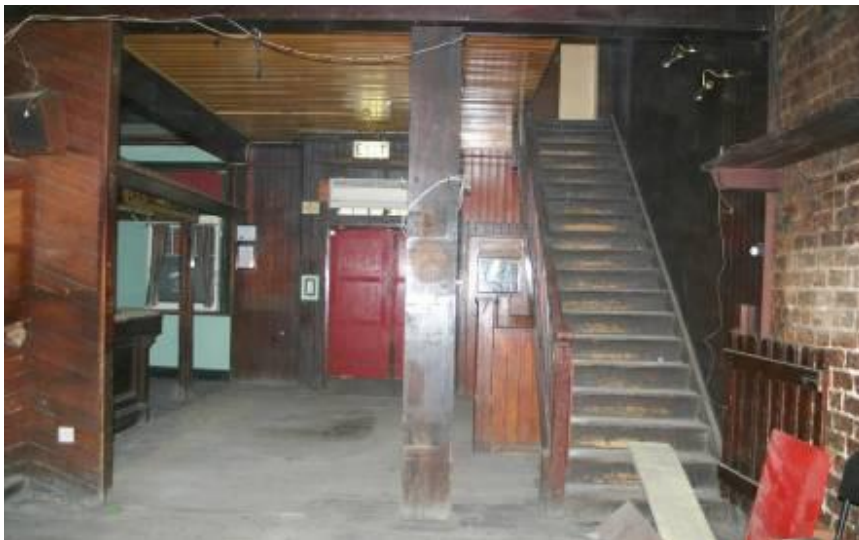
View of bar area towards front of building, showing stair to first floor.
