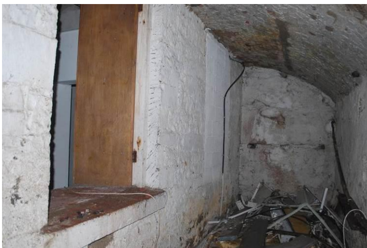
Fig. 2: Area to the front of the building below the footpath basement level.
