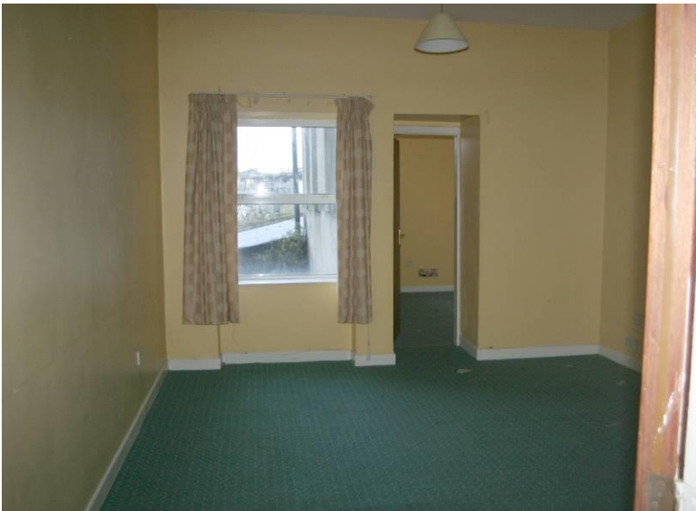
View of rear room, showing doorway through to the additional room to the rear located within the return (to first floor only).
