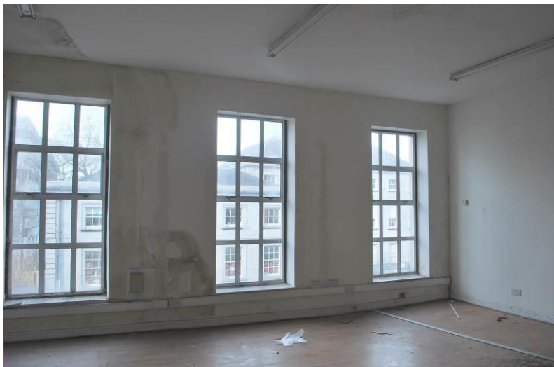
Fig. 1: Staining from water ingress visible to first floor, front room.
