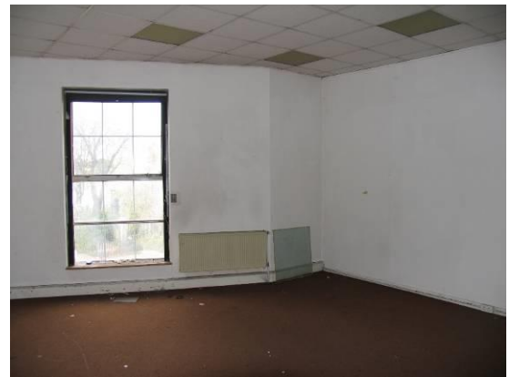
First floor facing front façade at location of kink in wall
