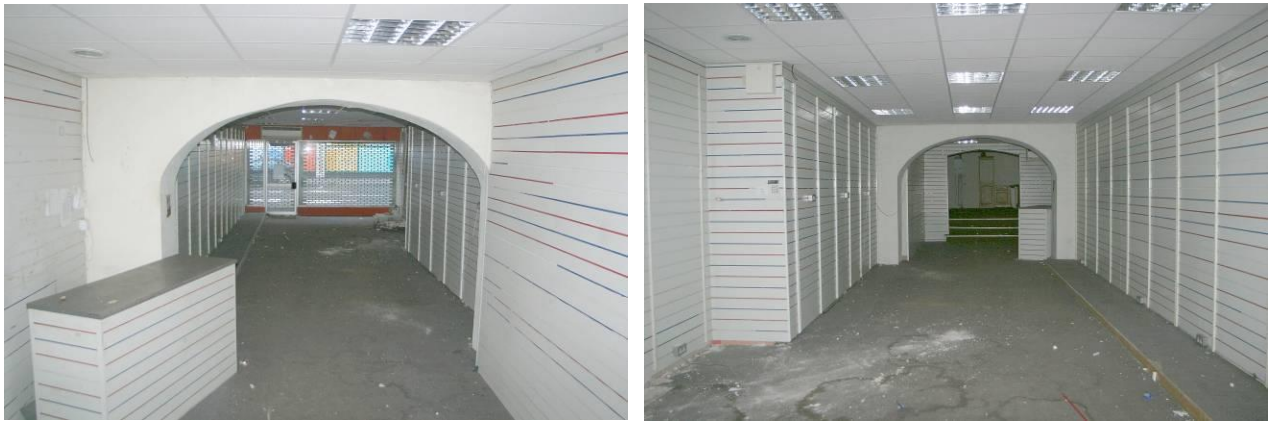
Views of the ground floor, towards the front of the building (above left) and to the rear (above right).
