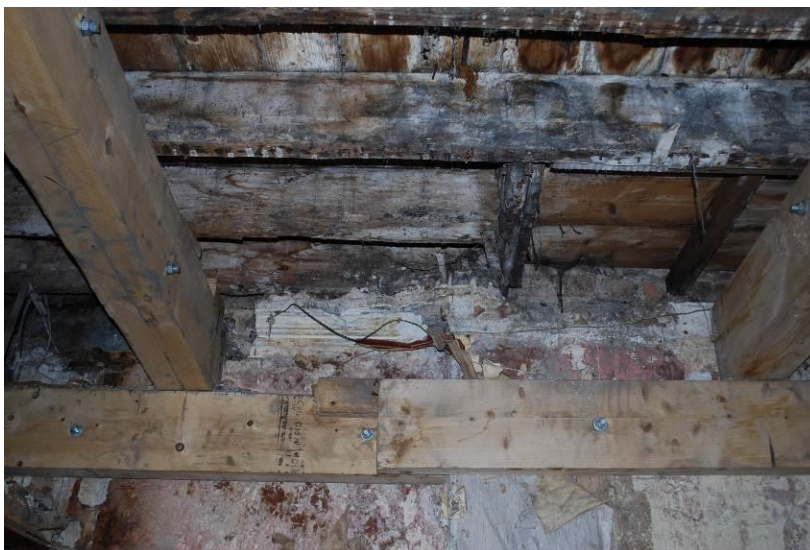
Fig. 4: Remnants of run plaster cornice, ground floor, previously hidden by later ceiling.
