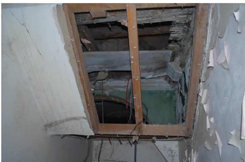
Fig. 2: Opening up works have revealed remnants of original plasterwork to
