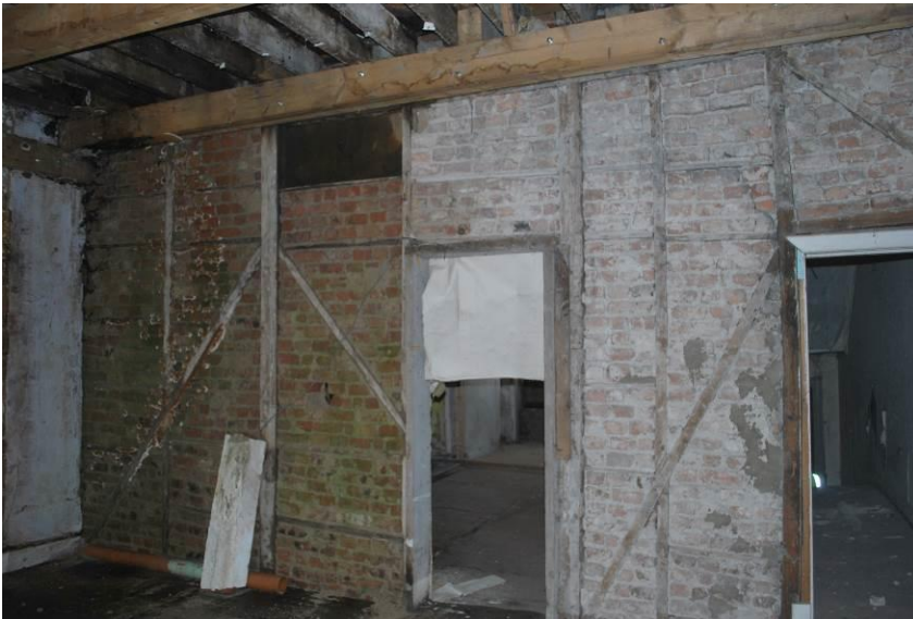
Fig. 3: Second floor, showing bricked nogged partition and water ingress along party wall.
