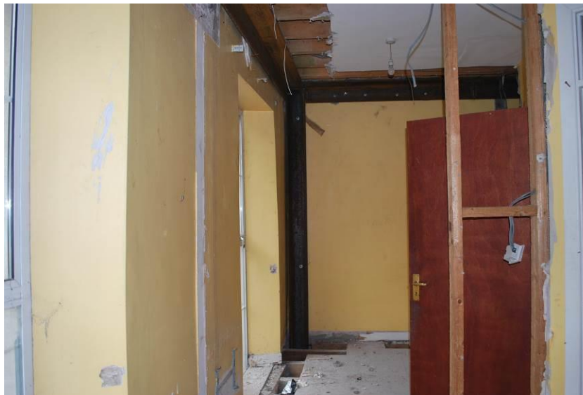
Fig. 2: First floor, front room, showing modern partitions and finishes, and remedial structural works.
