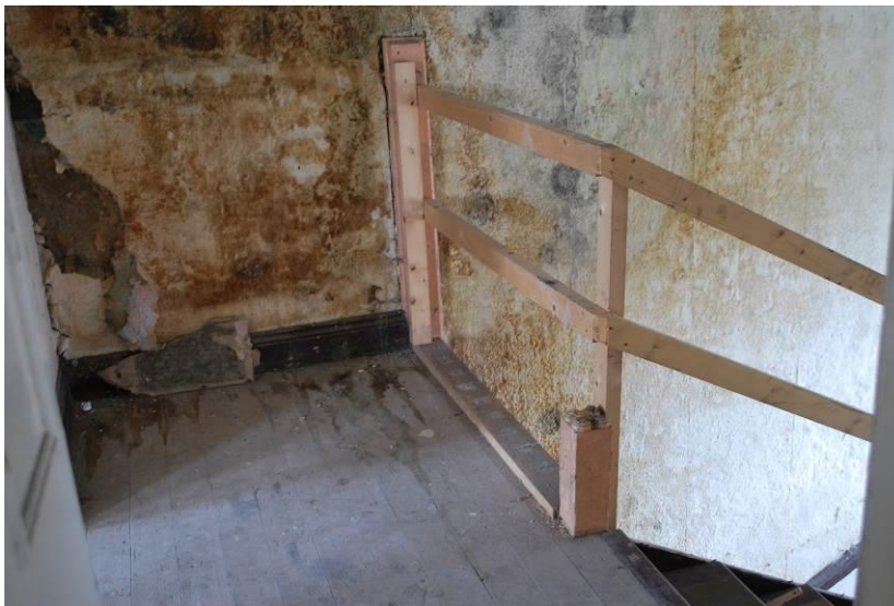
Fig. 5: Top landing with balustrade removed and broken newel post.
