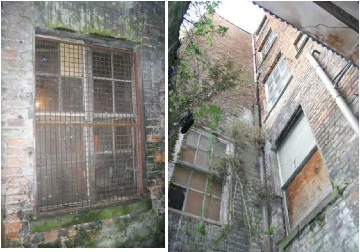
Rear elevation windows; at basement level (above left) and the remainder of the windows (above right).
