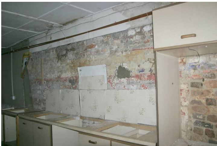
Area to the rear of the ground floor, within the adjoining building to the rear, showing brick walls.
