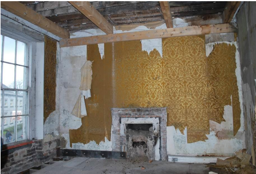
Fig. 1: First floor, front room, showing remedial structural works. The fire surround has been removed since this building was recorded in 2007.
