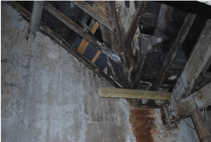
Fig. 1: Water ingress, top floor.
