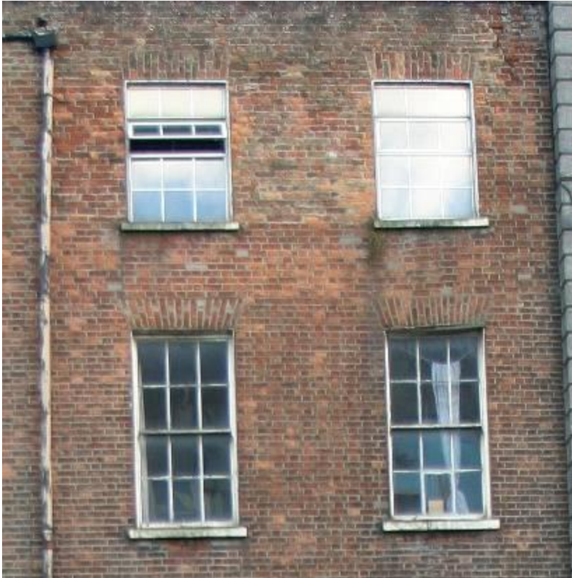
Detail of front elevation, showing timber replacement windows on the second floor, and uPVC to the third floor.
