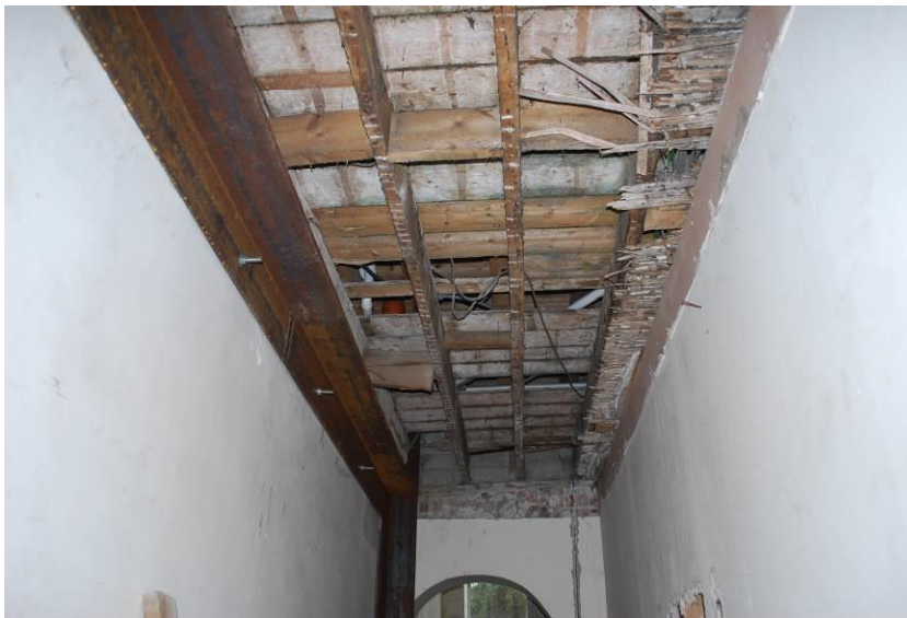
Fig 1: Steel beam inserted at ground floor level and ceiling removed to hall exposing remnants of historic timber floor and lath and plaster retained to this area of the building.
