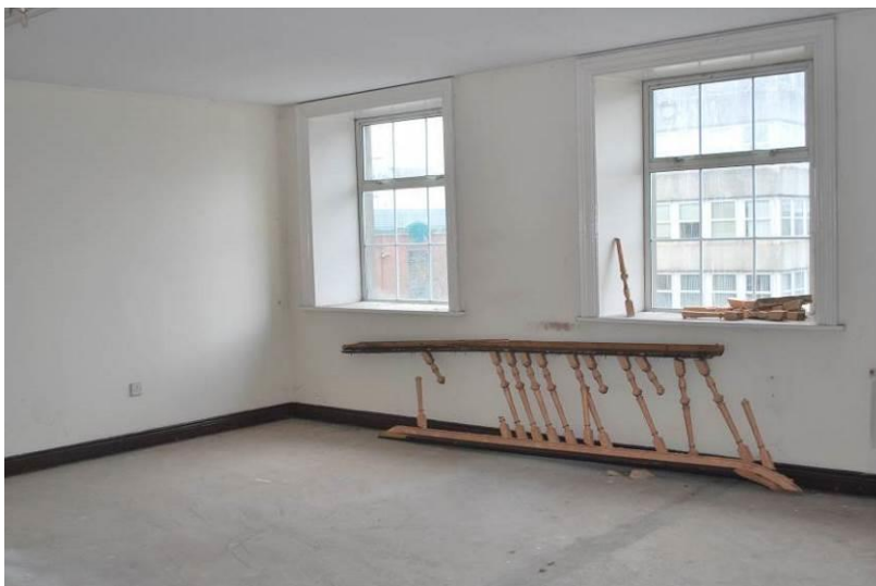
Fig. 7: Removed and damaged section of balustrade.
