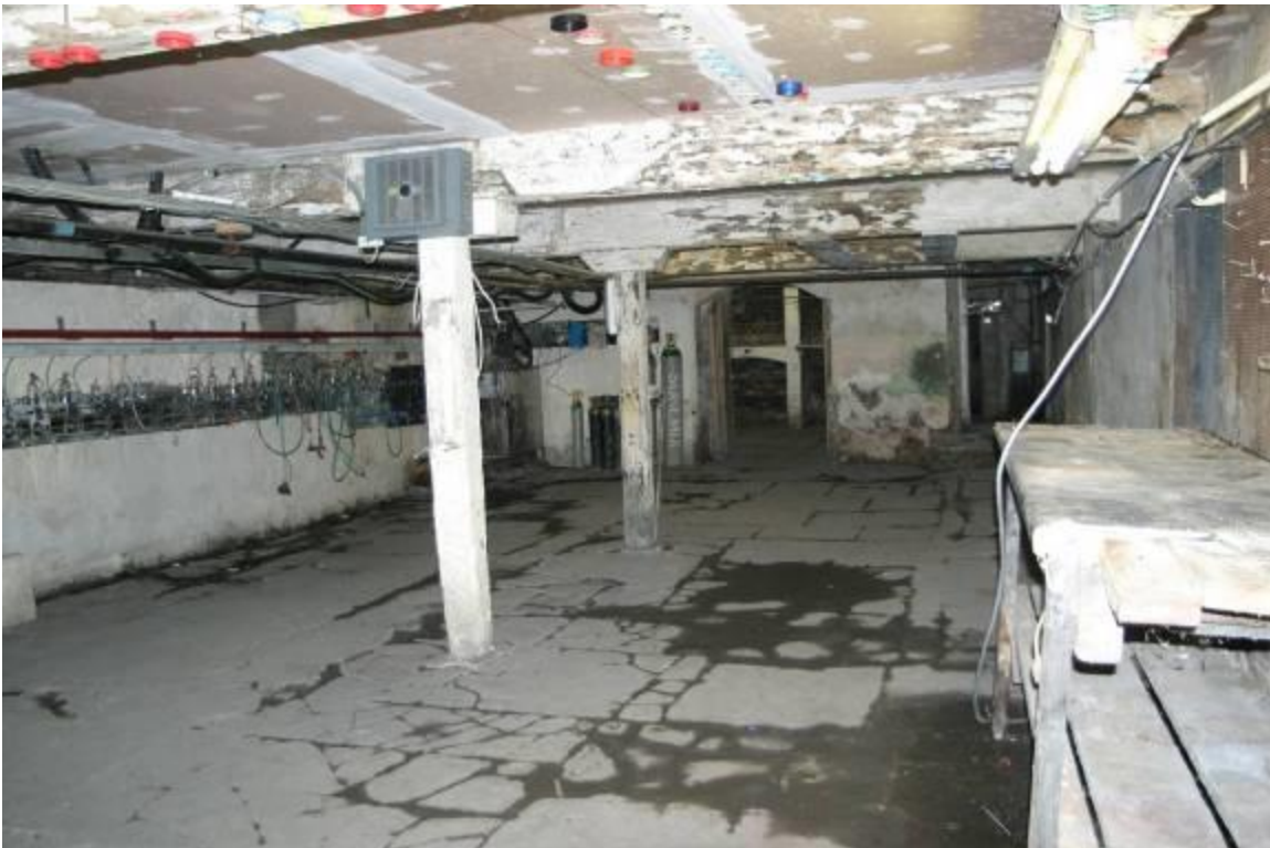
View of main basement area, from rear of building towards the front.
