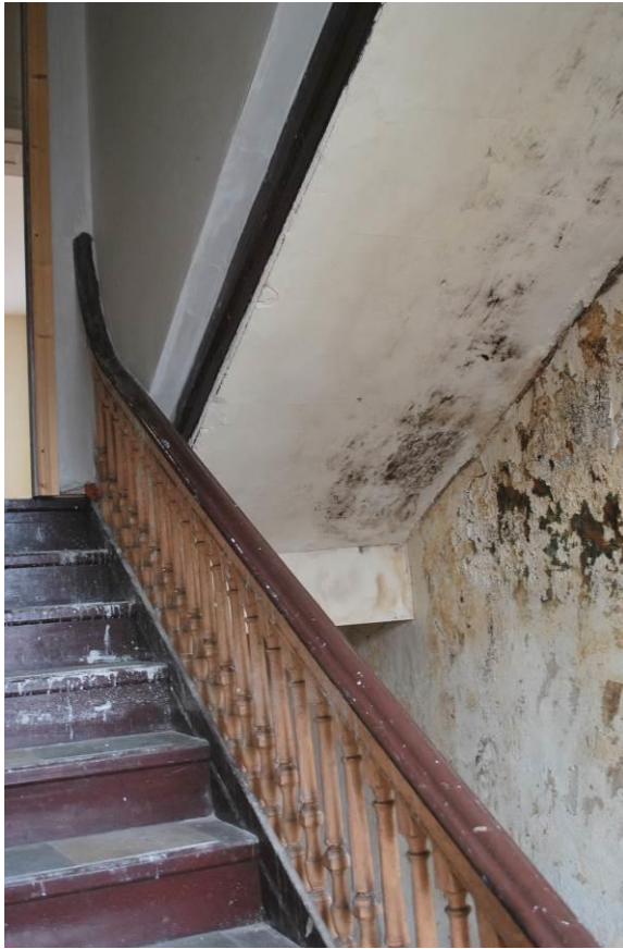
Fig. 3: Water ingress, party wall.
