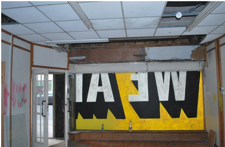
Fig. 1: Ground floor retail unit; sheeted timber ceiling retained above modern ceiling tiles.
