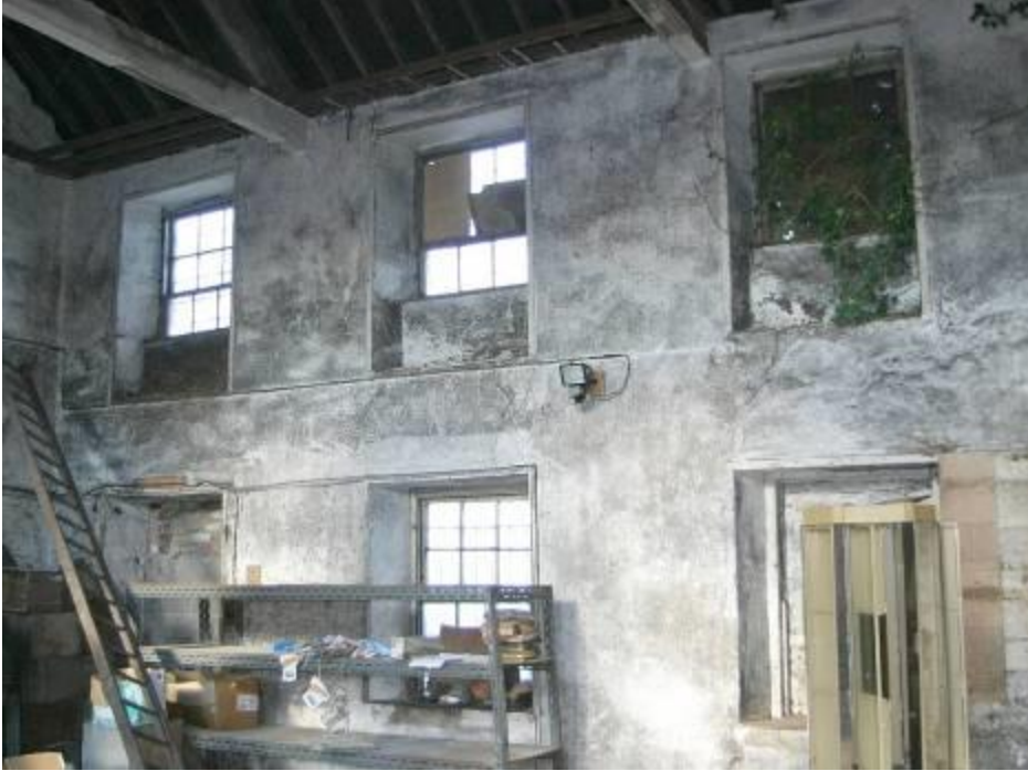
Windows to the rear elevation of the warehouse area (above garden world shop).
